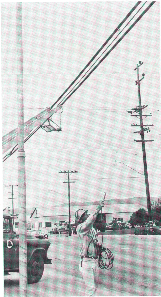
Ultrasonic detection of leaks in pressurized telephone cables has eliminated old-fashioned soap-bubble method. Leaks can usually be heard from the ground, often from a truck driving along the cable path. Translator responds only to sounds between 36 kHz and 44 kHz and is not affected by audible traffic noises.
